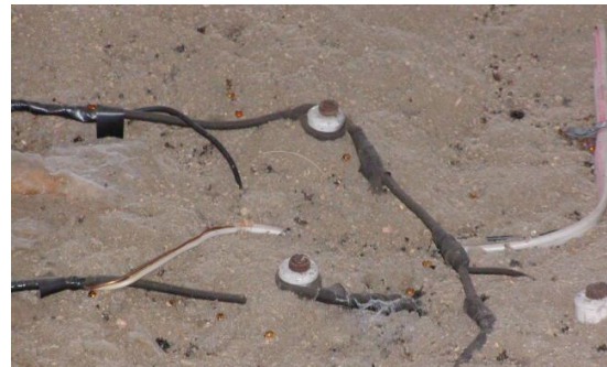
Note the improperly spliced wires buried in insulation. This photo shows a dangerous situation
